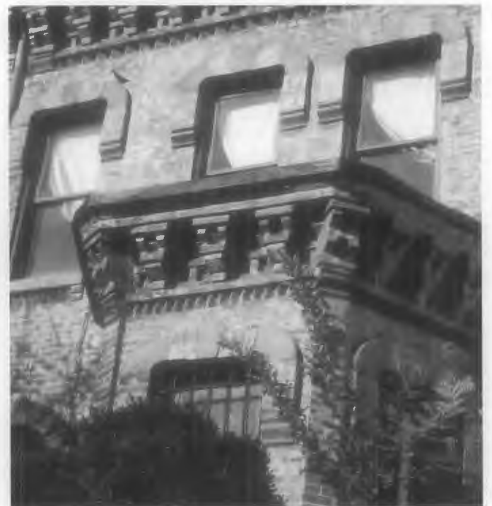
Figure 15. The whitish deposits left on the brick by a chemical paint remover may have resulted from inadequate rinsing or from the chemical being left on the surface too long and may be impossible to remove.
