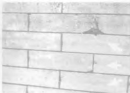
Figure 11. Rinsing with high-pressure water following chemical cleaning has left a horizontal line of abrasion across the bricks on this late-19th century row house.
