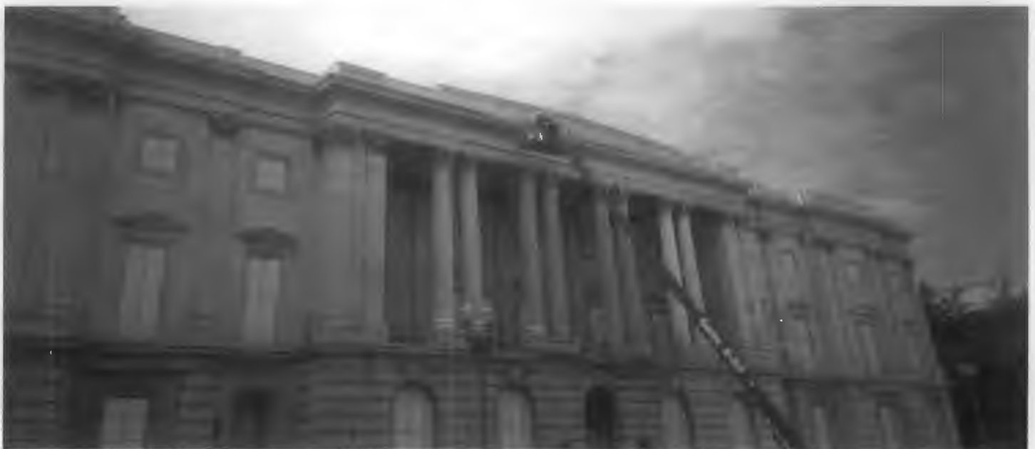
Figure 1. Low-to medium-pressure steam (hot-pressurized water washing), is being used to clean the exterior of the U.S. Tariff Commission Building, the first marble building constructed in Washington, D.C., in 1839. This method was selected by an architectural conservator as the "gentlest means possible" to clean the marble. Steam can soften heavy soiling deposits such as those on the cornice and column capitals, and facilitate easy removal. Note how these deposits have been removed from the right side of the cornice which has already been cleaned.
