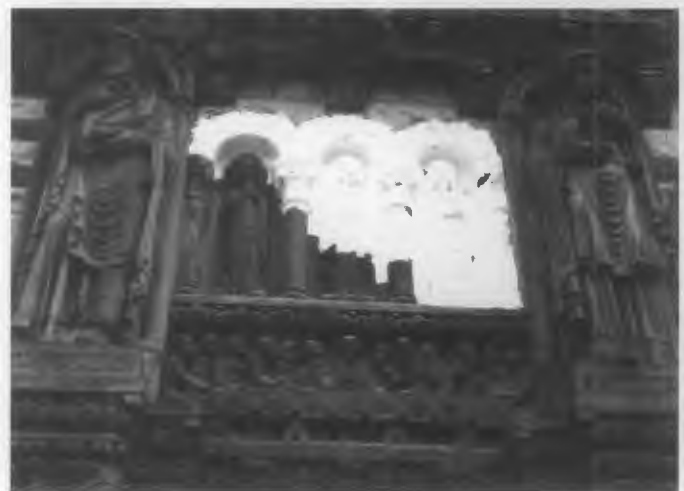
Figure 17. A poultice is being used to remove salts from the brownstone statuary on the facade of this late-19th century stone church. Photo: National Park Service Files.
