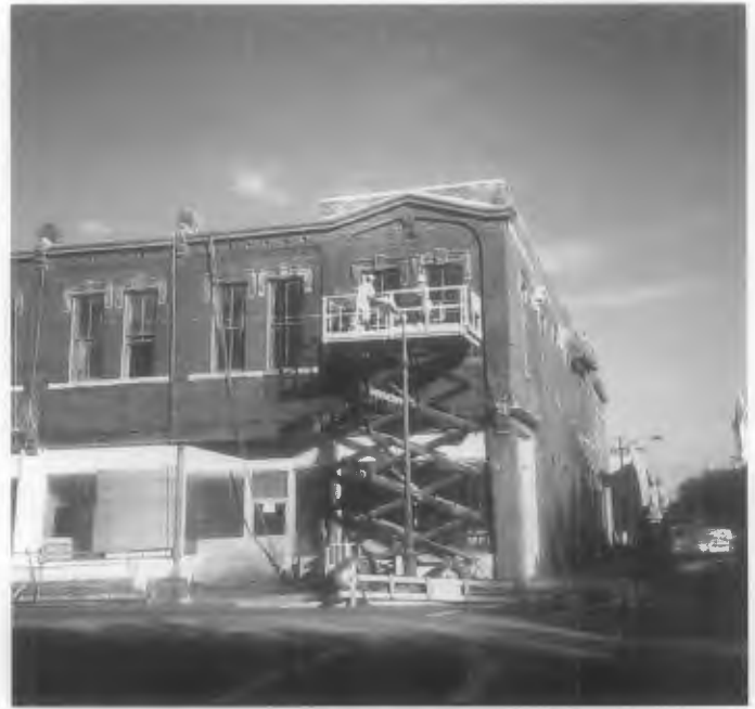
Figure 14. Chemical removal of paint from this brick building has revealed that the cornice and window hoods are metal rather than masonry.
