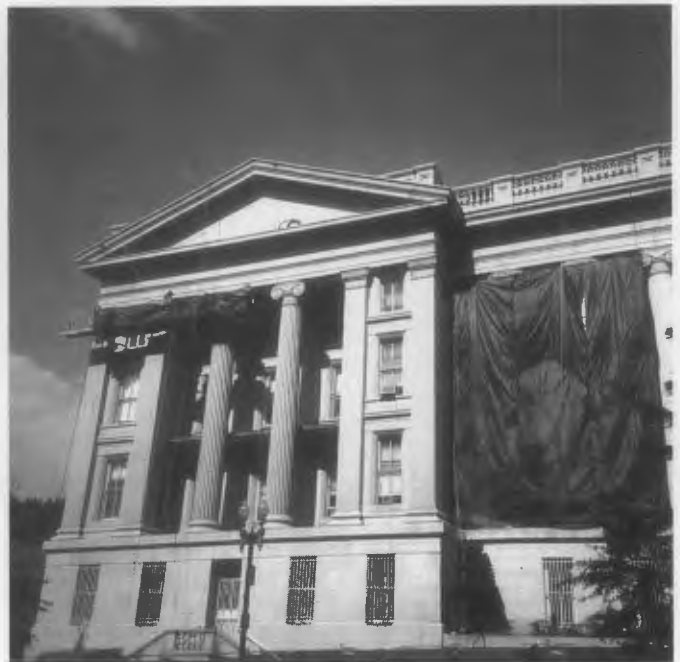
Figure 23. A tarpaulin protects and shields pedestrians from potentially harmful spray while chemical cleaning is underway on the granite exterior of the U.S. Treasury Building, Washington, D.C.
