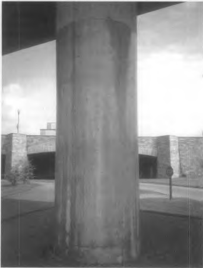
Figure 26. The anti-graffiti or barrier coating on this column is very shiny and would not be appropriate to use on a historic masonry building. The coating has discolored as it has aged and whitish streaks reveal areas of bare concrete where the coating was incompletely applied.
